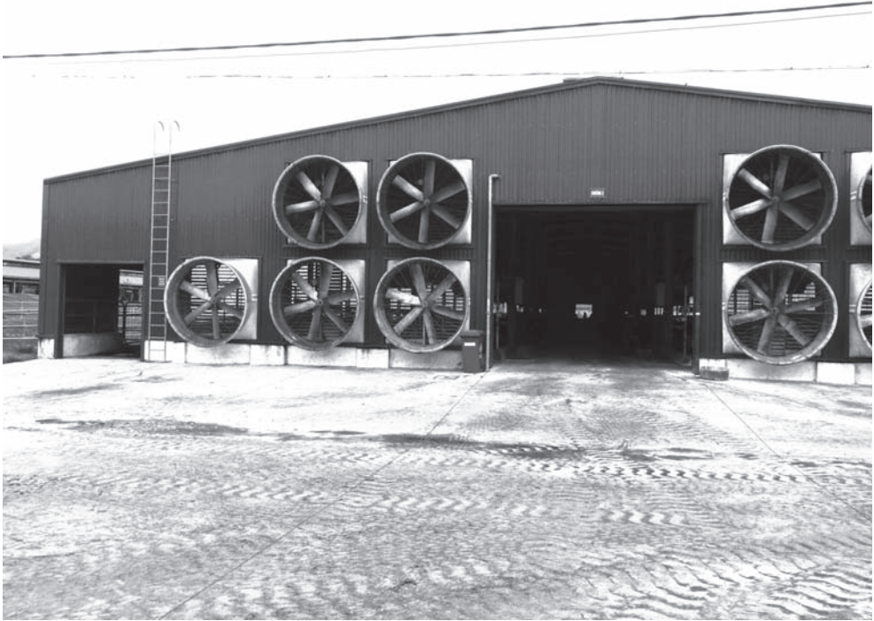
Figure 5.2: The tunnel ventilation shed would be considered an essential for any large-scale dairy feedlot in the humid tropics. It comprises a batch of large fans, as in this North Vietnam dairy feedlot. This shed has a second batch of fans at the other end of the shed, with one batch blowing and the second batch sucking, to produce a rapid air movement over the stock inside. In the dry tropics, ‘water curtains’ (or rubber strips over the fan outlets with water dripping off them) can be used to reduce air temperature but this system is ineffective in the humid tropics. The performance of high yielding cows in the lowland humid tropics will always be constrained for many months of the year by suppressed appetites which will reduce milk yields and increase the number of inseminations per conception. No matter what they cost, the tunnel ventilation shed must be considered a good investment. It is possible to modify non-ventilated sheds through a series of curtains along the sidewalls and baffles to direct the moving air over the cows.
